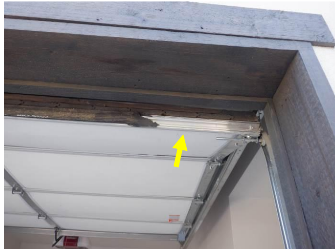
Photo 12: The bottom gaskets were damaged on both overhead garage doors (single door is shown).
