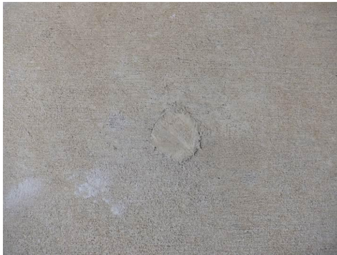
Photo 3: Patches in the patio slab were observed at approximately 10- to 12-foot intervals.
