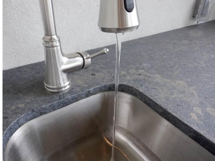
Photo 29: Water flow seemed very weak to this fixture.
