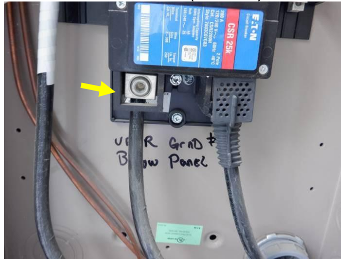
Photo 17: No barrier or cover was noted on one of the two service entrance terminals in the westernmost panelboard.
