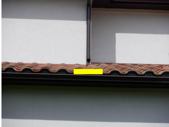
Photo 4: Splash guards were missing from the gutters in at least two locations on the rear (east) side of the roof over the patio.
