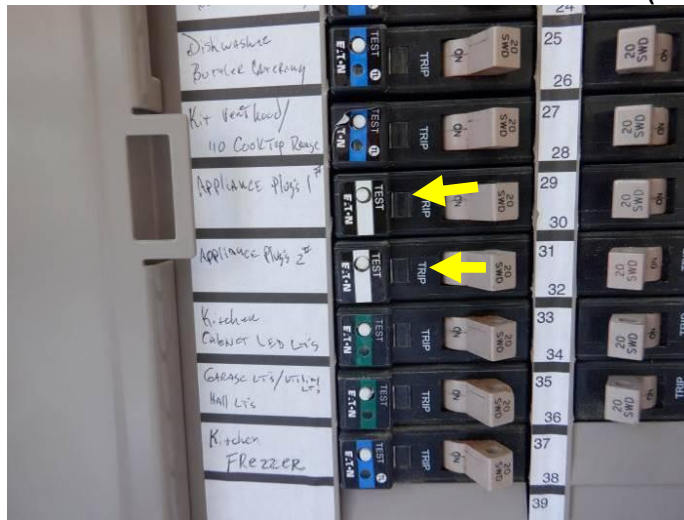
Photo 18: No arc-fault protection was noted for the two countertop appliance circuits for the kitchen counters, although GFCI protection was present.
