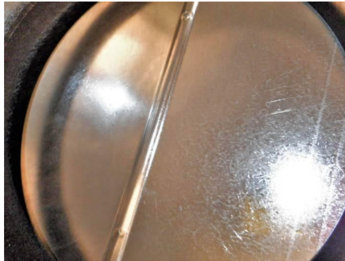
Photo A: The automatic damper did not open when the exhaust hood was activated on high speed (photo of the damper when the range vent was activated).
