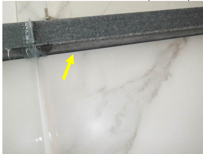
Photo 32: The caulking was incomplete beneath the shower bench.
