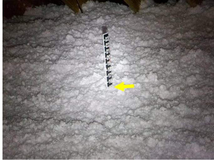
Photo 6: Lower areas of insulation were noted in the southeast portion of the uppermost attic.
