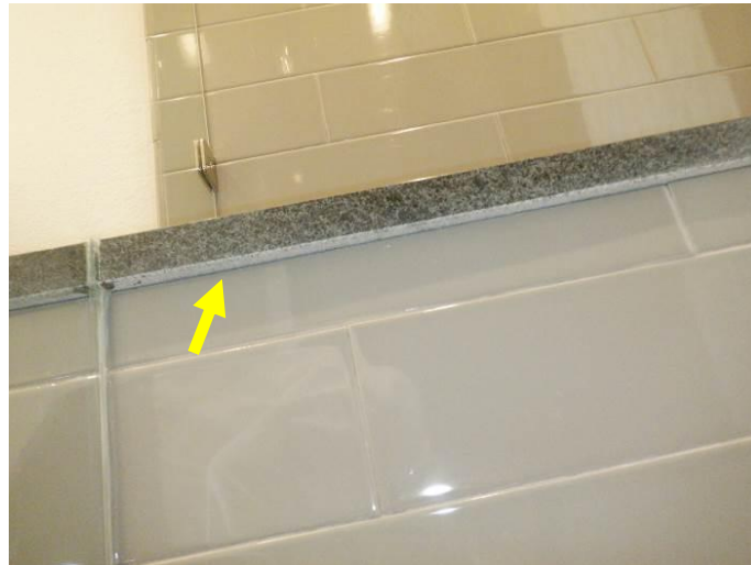
Photo 33: The underside of the bench and curb cap were not caulked (bench is shown).
