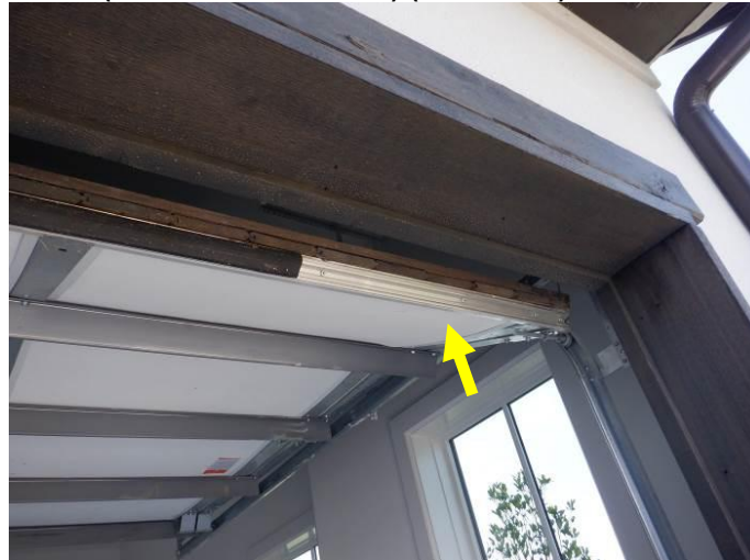
Photo 13: The bottom gaskets were damaged on both overhead garage doors (double garage door is shown).
