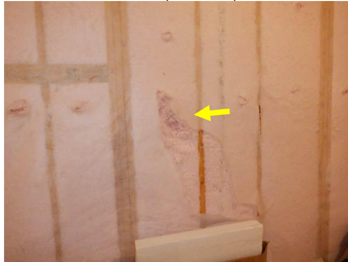
Photo 8: Some holes were noted in the insulation where exposed in the unfinished storage area.
