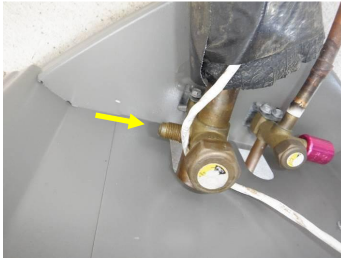
Photo 22: A safety cap was missing from the refrigerant line on the master bedroom condensing unit.
