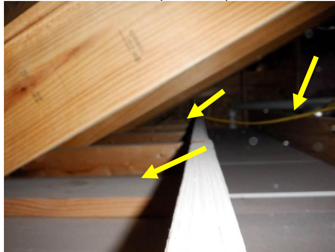
Photo C: No insulation was observed along the south perimeter of the attic space over the lower guest bathroom and closet as observed via camera from the temporary opening in the ceiling of the lower guest closet (west of the opening).
