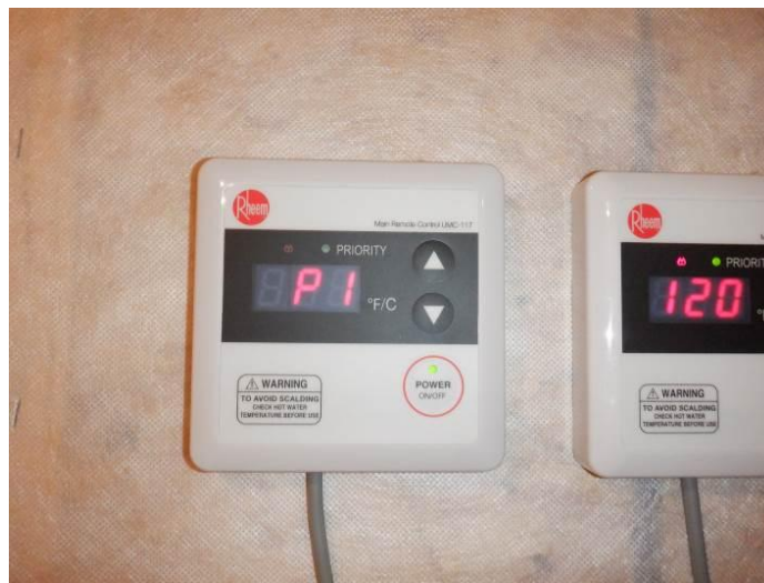
Photo 40: The water heaters would not remain activated and “P-1” codes flashed on both thermostat control pads (westernmost unit).
