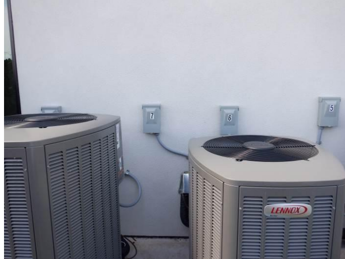
Photo 21: The services disconnect panels for two exterior condensing units were located behind the condensing units.
