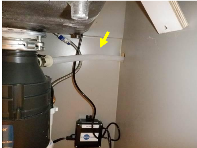
Photo 42: No adequate anti-siphon loop or air gap fixture was present in the dishwasher drain line in the butler's pantry.
