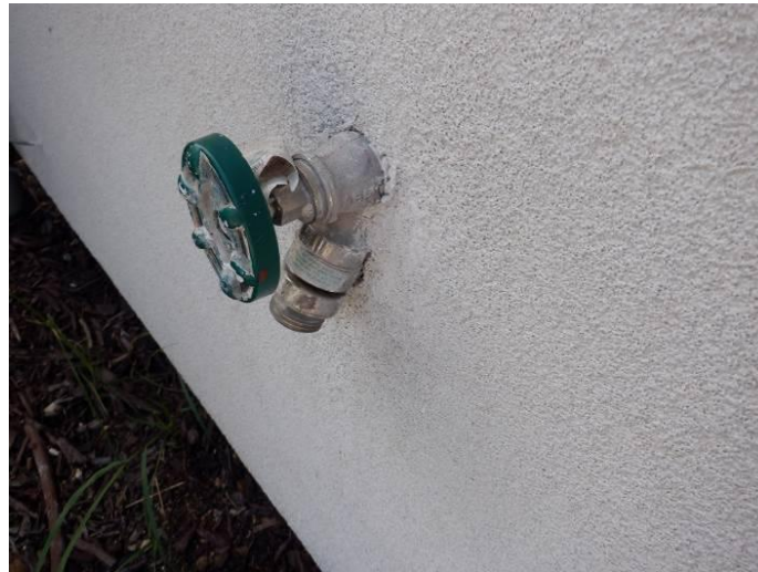
Photo 36: All exterior faucets were embedded into the stucco (north side is shown).
