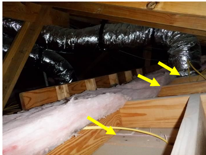
Photo B: No insulation was observed along the south perimeter of the attic space over the lower guest bathroom and closet as observed via camera from the temporary opening in the ceiling of the lower guest closet (east of the opening).
