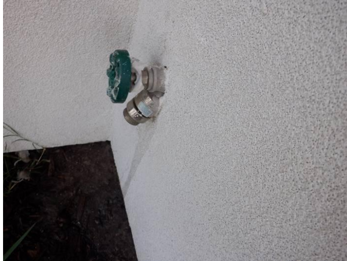
Photo 37: All exterior faucets were embedded into the stucco (west side is shown).
