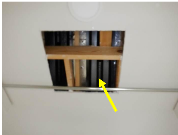
Photo D: A temporary opening was observed in the ceiling of the guest bathroom closet.
