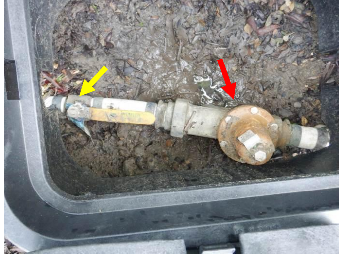
Photo 27: The water supply shutoff valve for the house (yellow arrow) along with a pressure-reducing valve (PRV) (red arrow) was located in the valve box in the front beds.
