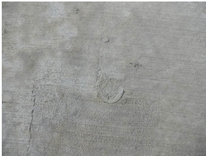
Photo 1: Patches in the patio slab were observed at approximately 10- to 12-foot intervals.
