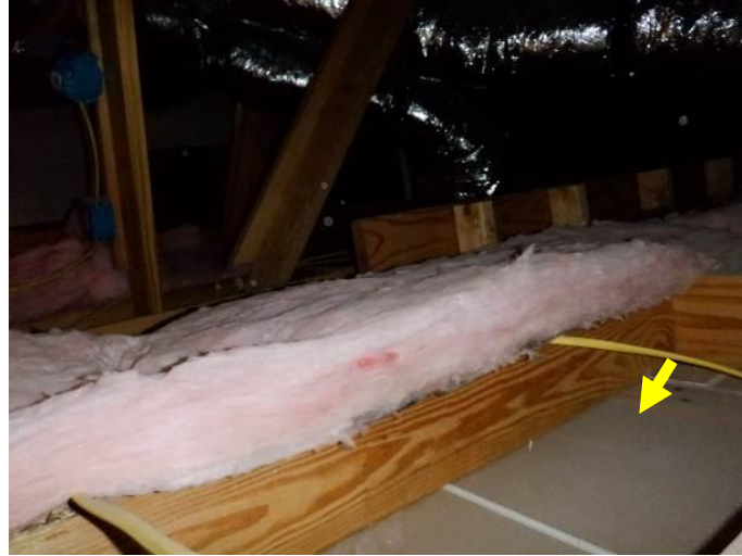
Photo A: No insulation was observed along the south perimeter of the attic space over the lower guest bathroom and closet as observed via camera from the temporary opening in the ceiling of the lower guest closet (at the access opening).
