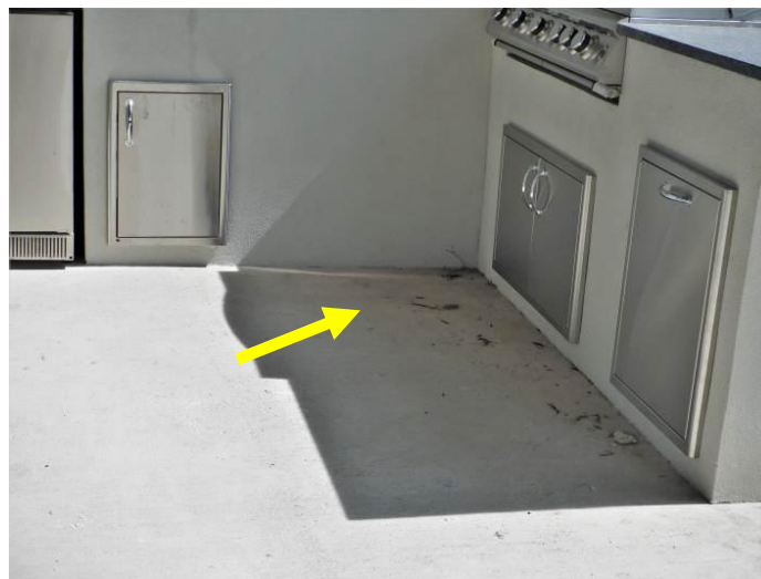
Photo 16: A water entrapment condition was noted at the outdoor kitchen area.
