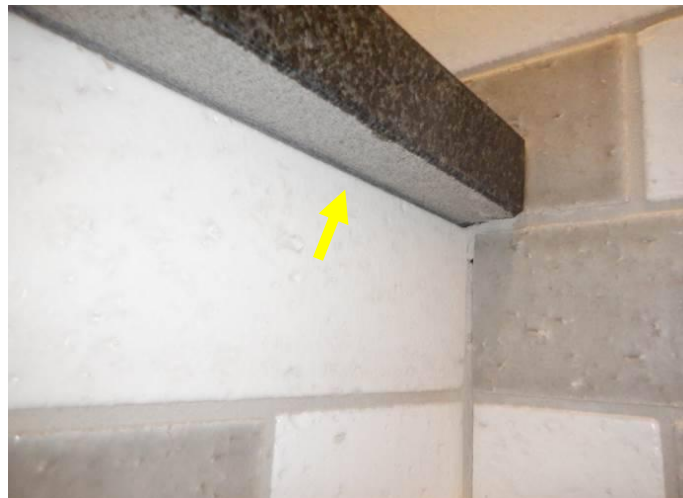
Photo 35: The undersides of the bench and the curb cap were not caulked (shower bench is shown).
