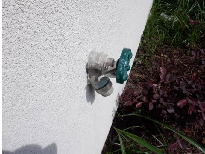
Photo 38: All exterior faucets were embedded into the stucco (north side is shown).
