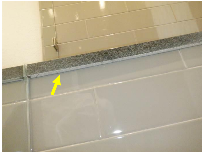
Photo 33: The underside of the bench and curb cap were not caulked (bench is shown).
