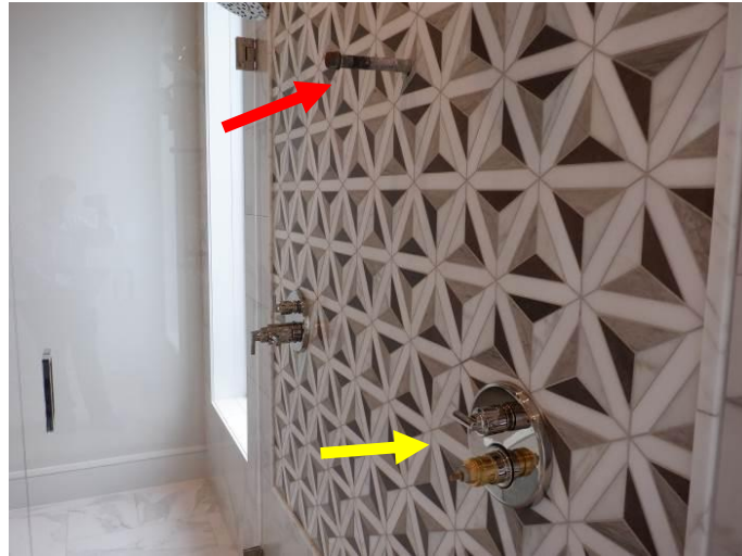
Photo 30: The easternmost shower valve installation was incomplete (yellow arrow). The wand fixture for the westernmost shower diverter was not installed (red arrow).
