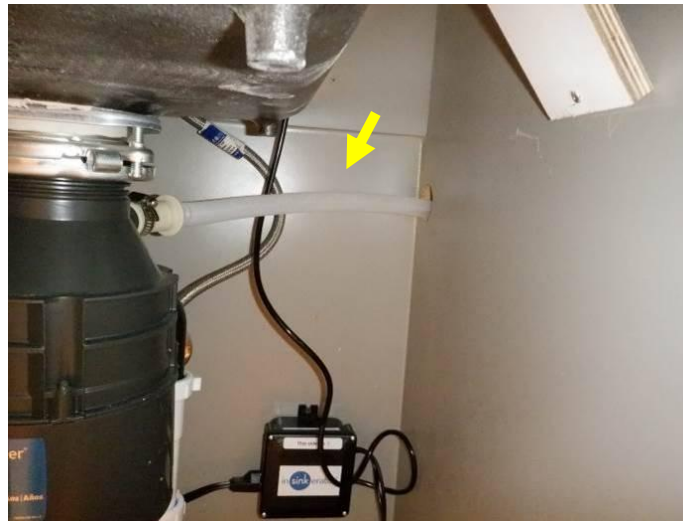
Photo 42: No adequate anti-siphon loop or air gap fixture was present in the dishwasher drain line in the butler's pantry.
