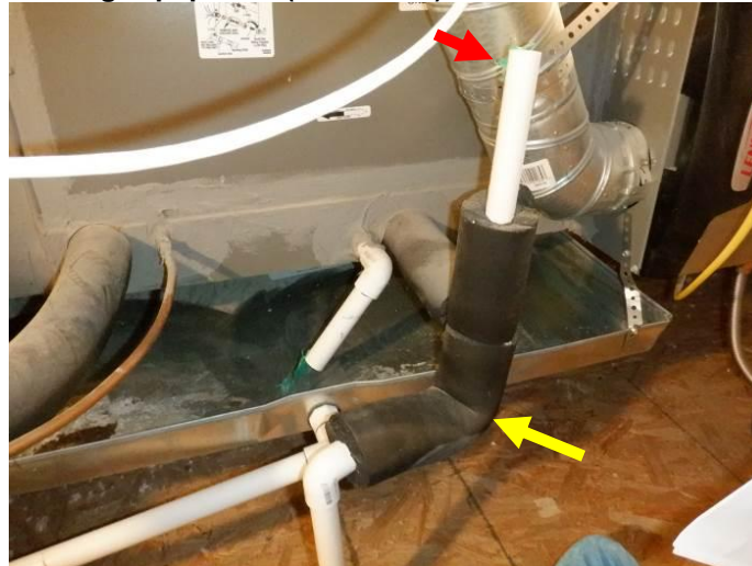
Photo 24: The P-trap (yellow arrow) was installed on the downstream side of the vent pipe (red arrow) for the primary condensate drain line of each HVAC system (master bedroom unit is shown).
