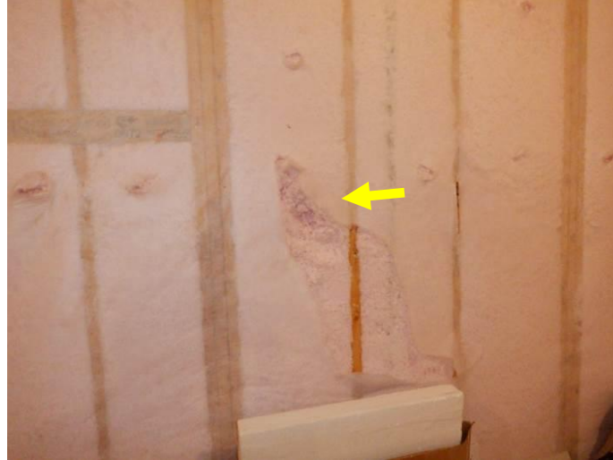
Photo 8: Some holes were noted in the insulation where exposed in the unfinished storage area.
