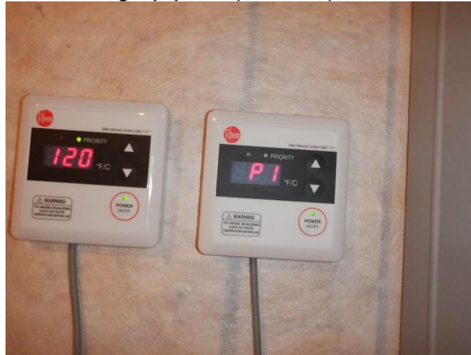
Photo 41: The water heaters would not remain activated and “P-1” codes flashed on both thermostat control pads (easternmost unit).
