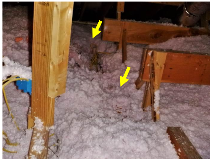
Photo 7: Lower areas of insulation were noted in the southeast portion of the uppermost attic.
