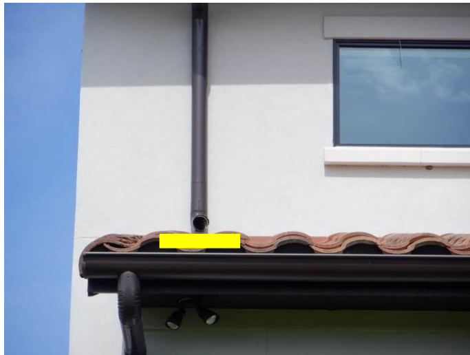
Photo 5: Splash guards were missing from the gutters in at least two locations on the rear (east) side of the roof over the patio.
