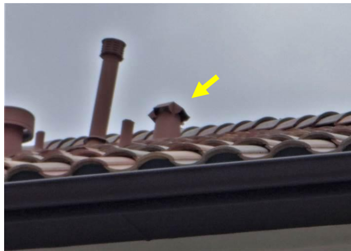
Photo 45: The exhaust duct discharged through an exhaust terminal without a backdraft damper.
