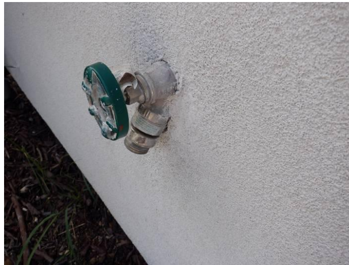
Photo 36: All exterior faucets were embedded into the stucco (north side is shown).
