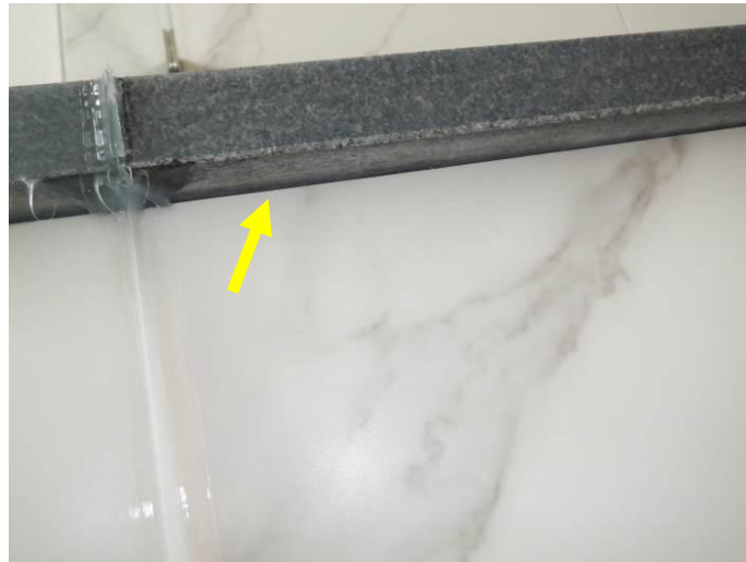
Photo 32: The caulking was incomplete beneath the shower bench.
