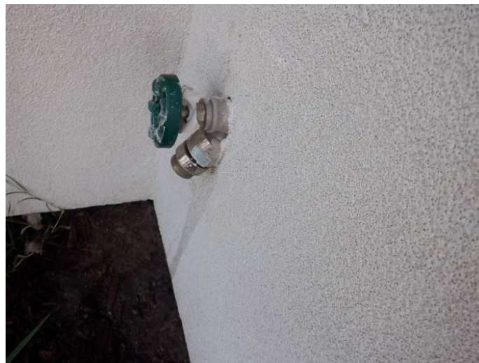
Photo 37: All exterior faucets were embedded into the stucco (west side is shown).
