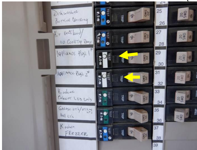
Photo 18: No arc-fault protection was noted for the two countertop appliance circuits for the kitchen counters, although GFCI protection was present.
