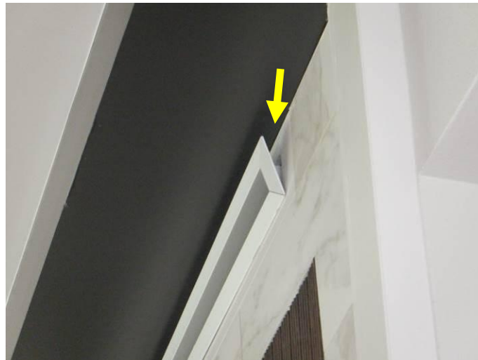
Photo 15: The trim kit for the fireplace blower was not secured.
