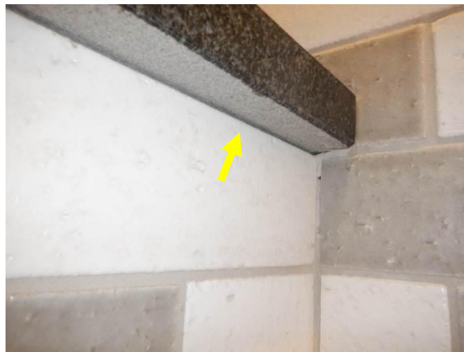
Photo 35: The undersides of the bench and the curb cap were not caulked (shower bench is shown).
