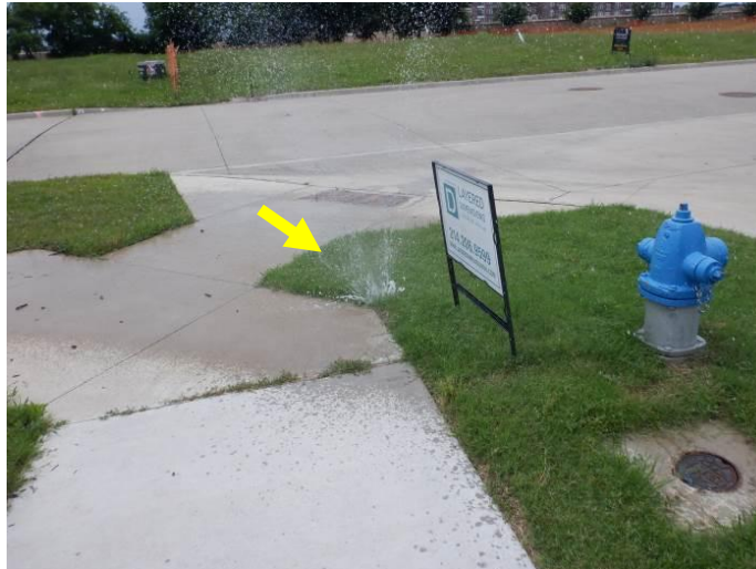
Photo 46: At least one leak was noted at the south end of the parkway.
