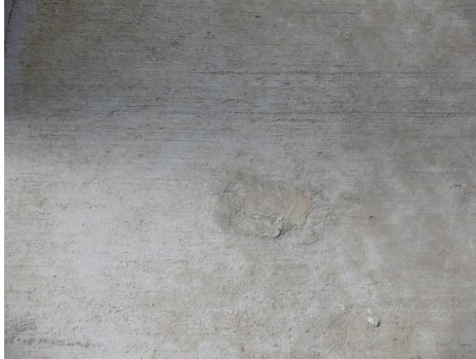
Photo 2: Patches in the patio slab were observed at approximately 10- to 12-foot intervals.
