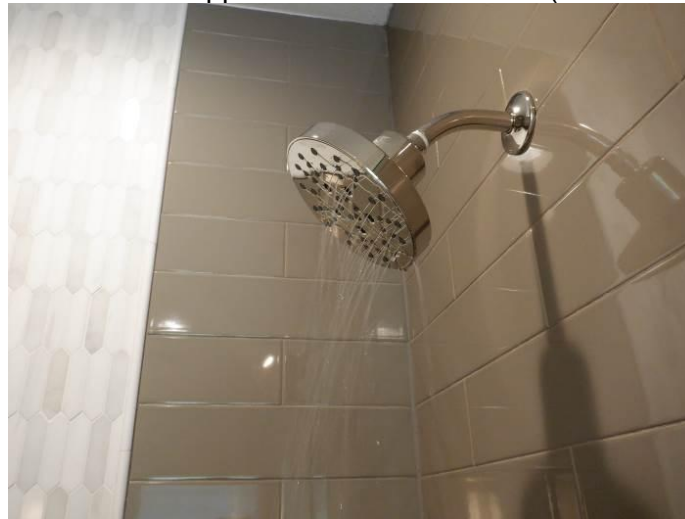
Photo 34: Very poor water flow was noted at the shower head.
