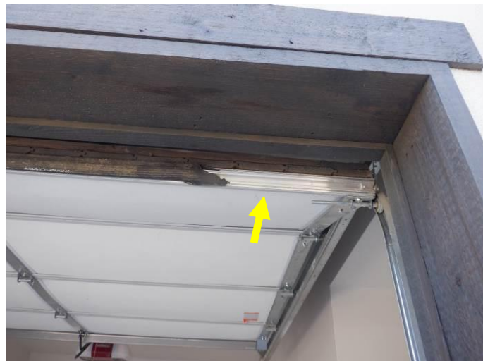
Photo 12: The bottom gaskets were damaged on both overhead garage doors (single door is shown).
