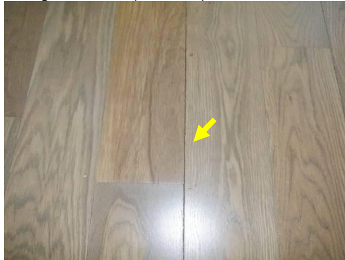
Photo 10: A noticeable gap was noted in the wood flooring in at least one location in the upper hall.
