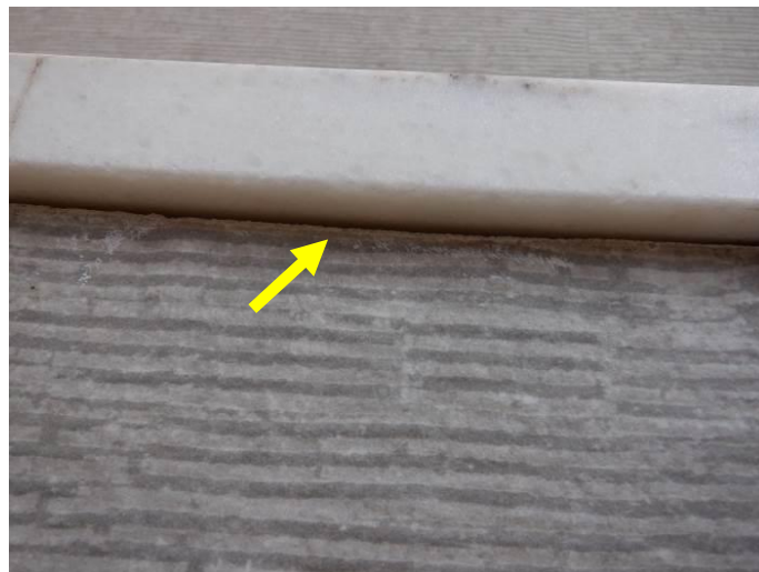
Photo 31: The caulking was incomplete beneath the shower bench. (Continued)
