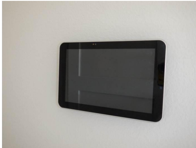
Photo 20: The thermostat for this system was found blank and unresponsive.
