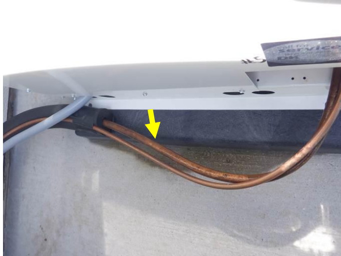
Photo 23: A portion of the suction line insulation was missing from the Emerson condensing unit
