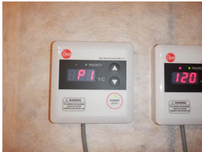
Photo 40: The water heaters would not remain activated and "P-1" codes flashed on both thermostat control pads (westernmost unit).
