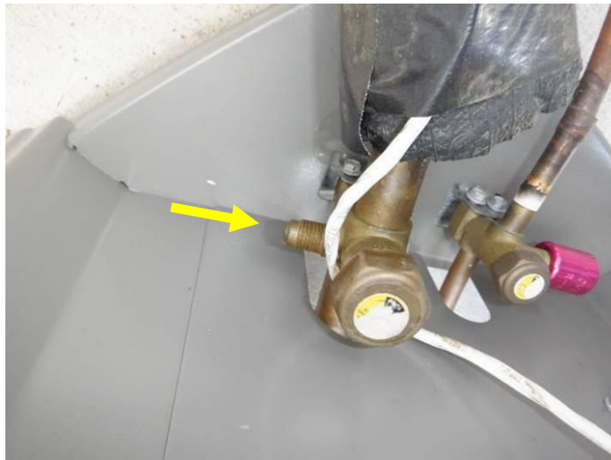
Photo 22: A safety cap was missing from the refrigerant line on the master bedroom condensing unit.
