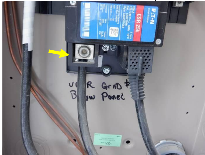
Photo 17: No barrier or cover was noted on one of the two service entrance terminals in the westernmost panelboard.
