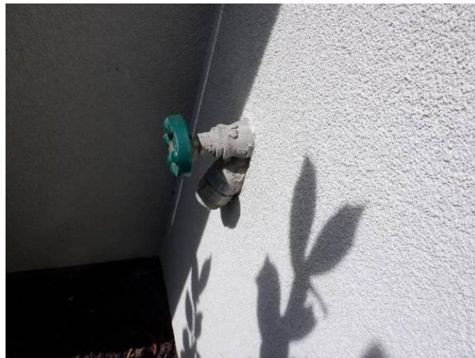
Photo 39: All exterior faucets were embedded into the stucco (east side is shown).
